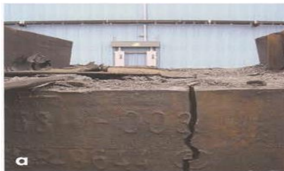
Figure 1 the fractured base before repair
