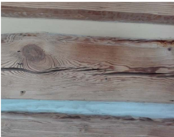
Figure 5. Painting of the joints: upper joint after painting, bottom joint prior to being painted
